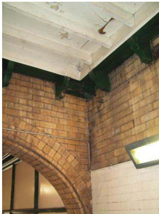
Photo A. Cracked conduit in Booking Hall ceiling which drips heavily during rain.
